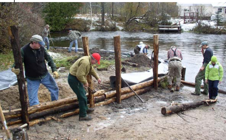
Members from Paul Young and Mason-Griffith Founders Chapters of Trout Unlimited along with Huron Pines staff repair the Wakeley Bridge Landing. Erosion resulting from parking lot runoff created a gully to the river. In addition to the stream stabilization, partners made the site handicap accessible. Funding for the site work was provided by Crawford County.
