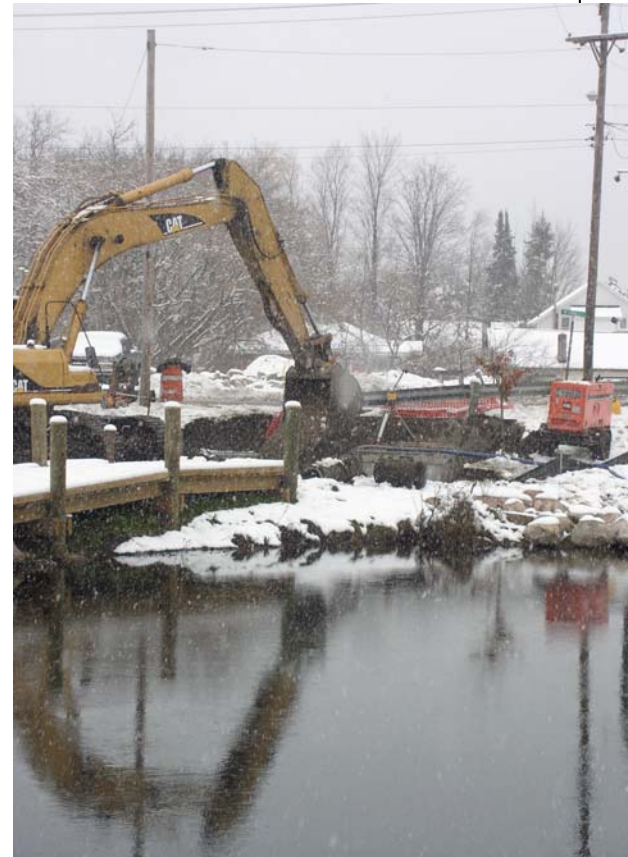
November 2006 installation of a stormwater oil-grit separator in Grayling to reduce pollution that harms the Au Sable River.
