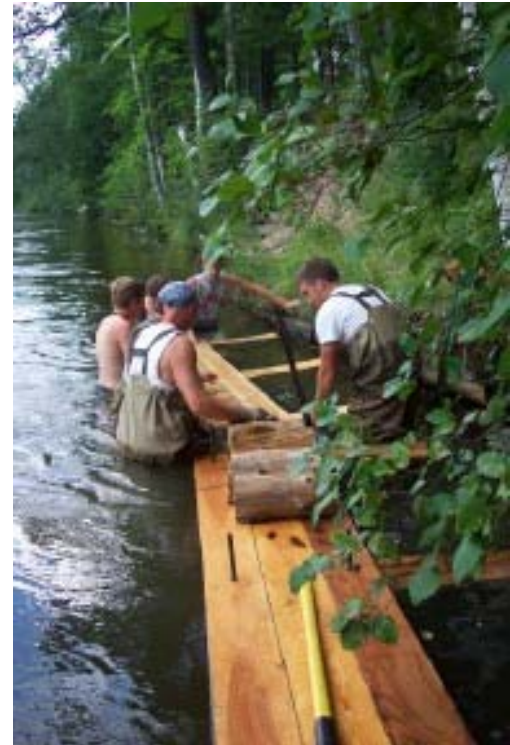
Above: Members of the Restoration Crew install a LUNKER structure on the Au Sable River. LUNKER structures serve two purposes: to control erosion by stabilizing the toe and bank of the river and to provide habitat for fish and other aquatic animals.
