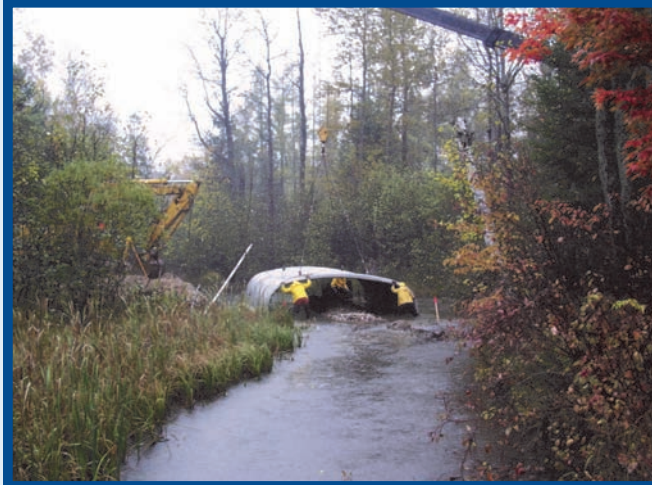
The Otsego County Road Commission replaced a culver on Crapo Creek to reduce sediment runoff and improve fish habitat.
