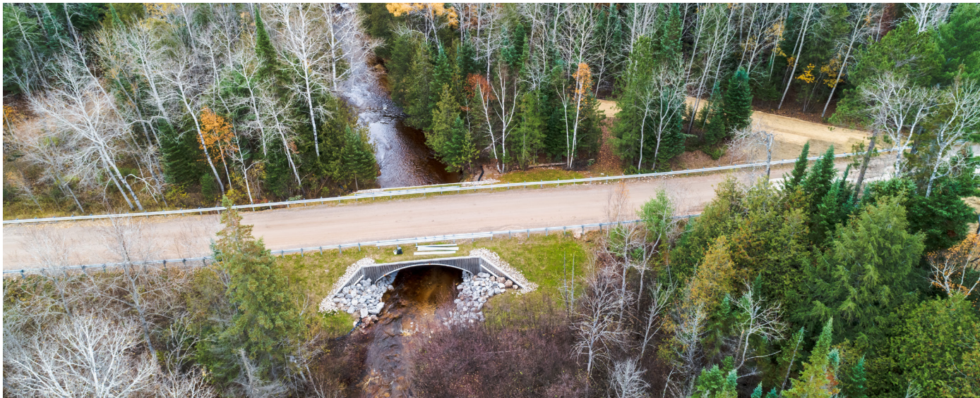
Water runs freely under the new Waveland Rd. crossing over Milligan Creek. The final touches on the project will conclude this spring when the roads are resurfaced with asphalt to prevent excess sediment from entering the water. Photos: Tom Cadwalader
