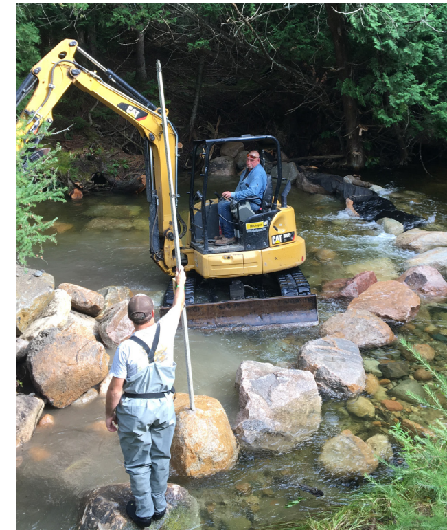
Boulders being placed in the South Branch River to increase water levels.
