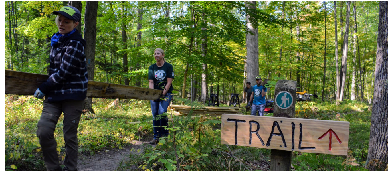
Andrea Foster of The Little Forks Conservancy (left) and Jennie Zoll of Huron Pines carry a timber beam for a new footbridge at a Midland nature preserve.
