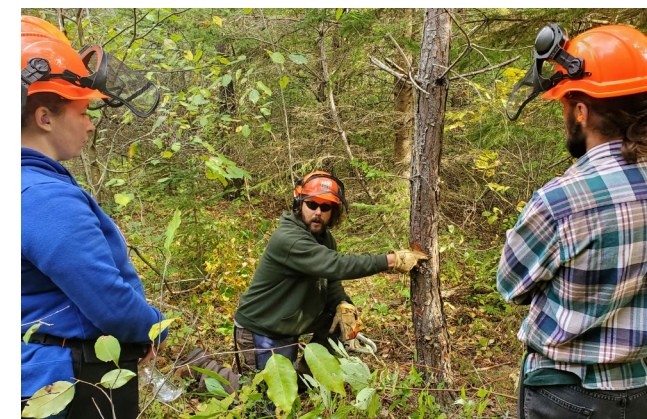
Conservation Stewardship Director Steve Woods gives staff instruction on chainsaw operation to remove invasive Scotch pine as part of Duncan Bay wetland restoration.
