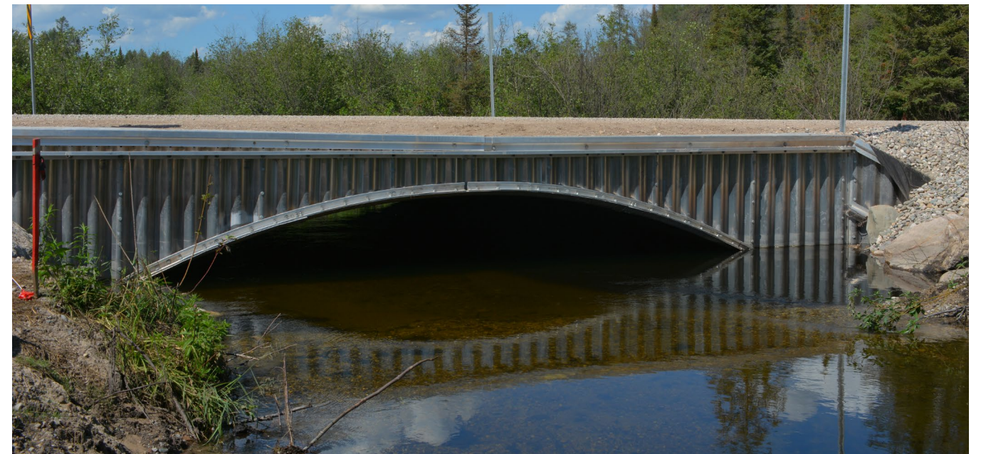
The finished product which restores a more natural flow to the East Branch Black River and connects trout to 20 miles of upstream habitat.
