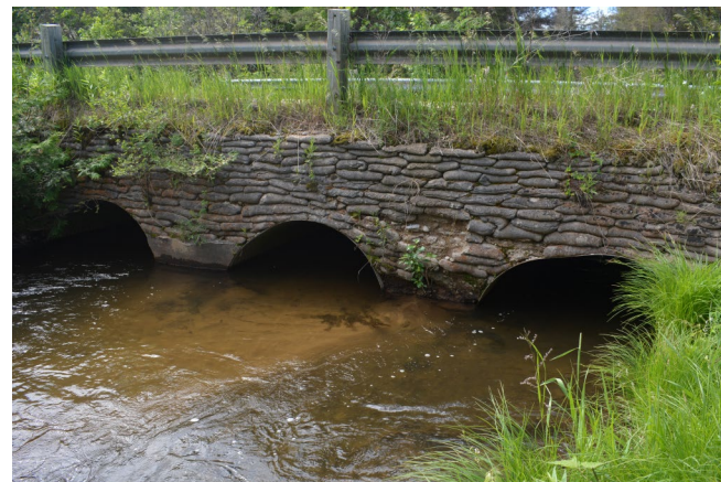
Gilchrist Creek at Harwood Road consisted of three undersized culverts, restricting river flow and fish movement.
